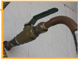
Cold water inlet valve
