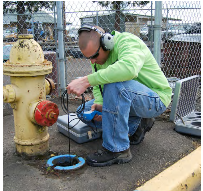
Water Foreman Jason Owens uses survey equipment to listen for a water leak. Customers may see SUB crews at hydrants and water meters hunting down subterranean leaks.
