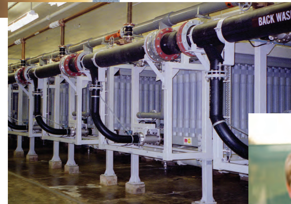
A membrane filter system in action.
